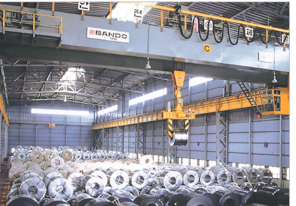
:: COIL 운반용 CRANE(COIL LIFTER) ::
